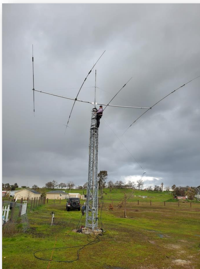
Vina K6VNA (up tower) and Dennis NJ6G, performing antenna repairs between rain showers during recent storms.
